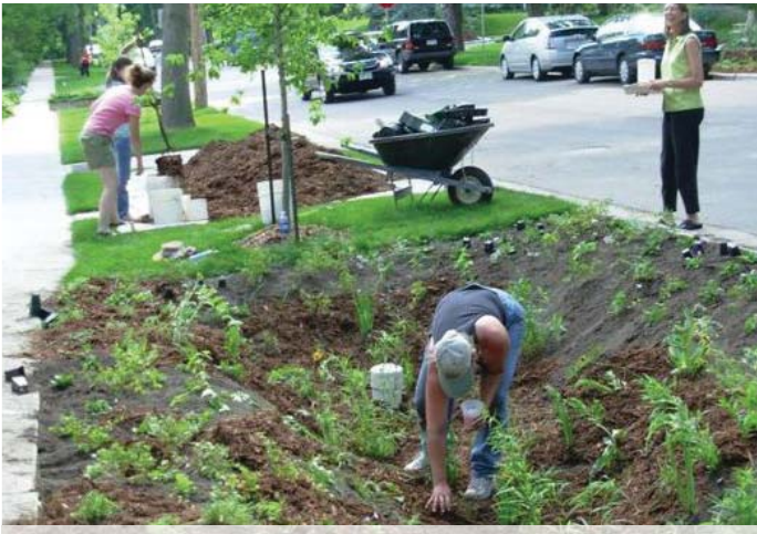
Figure 5.7: Bio-filtration swale - Madison WI, USA
