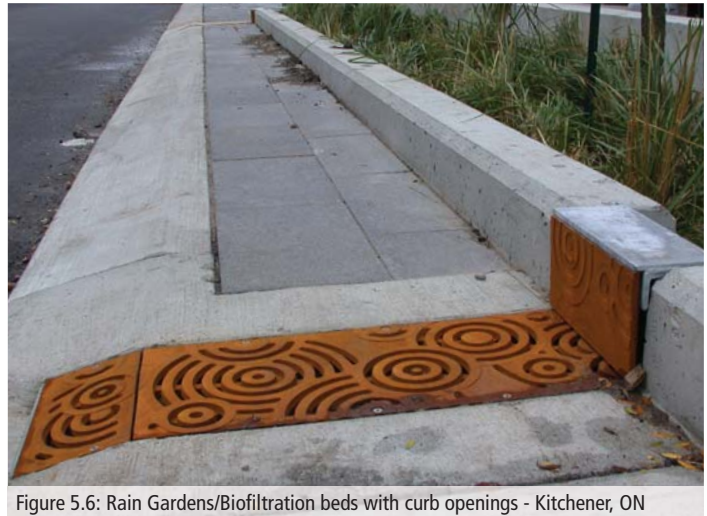
Figure 5.6: Rain Gardens/Biofiltration beds with curb openings - Kitchener, ON
