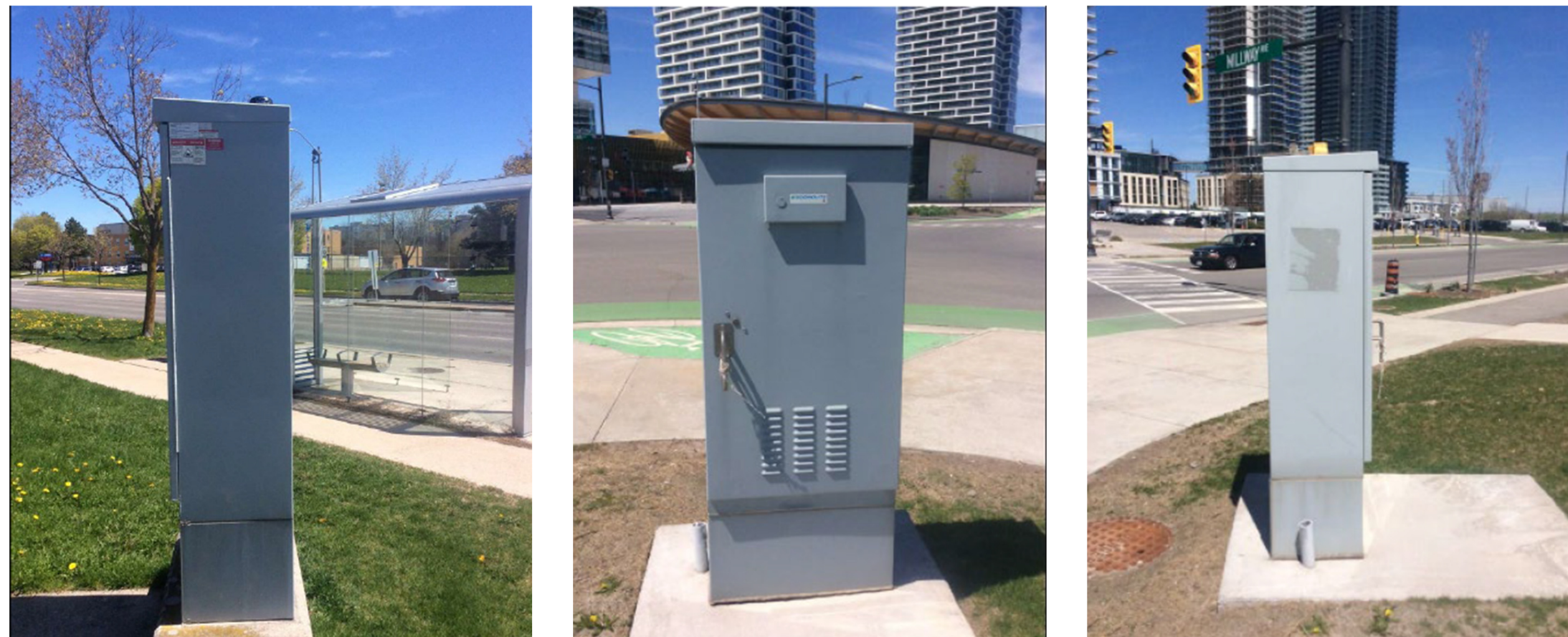
Example Traffic Signal Cabinets
